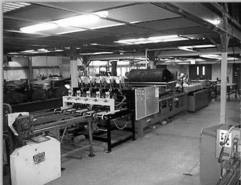
The complete coil line with the new equipment installed is 7 feet shorter than before the new equipment was added.
